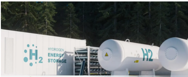
Fig. 20 Hydrogen Energy storage [36]
